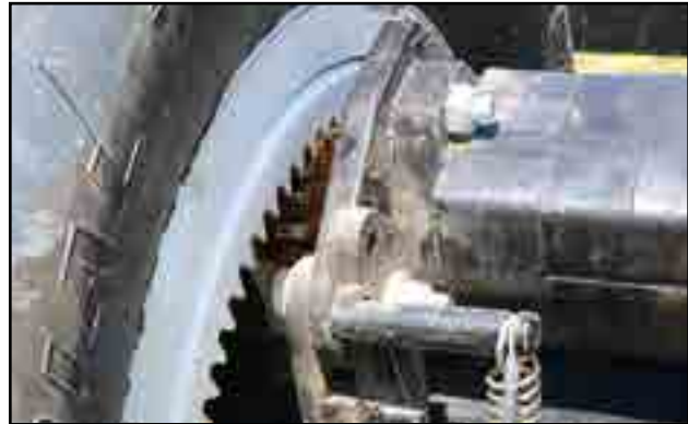
Fig 110 - Bin fill conveyor drive gears
