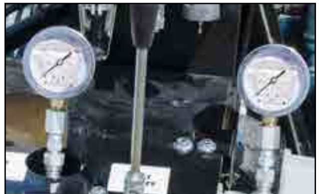
Fig 14 - Hydraulic pressure gauges
