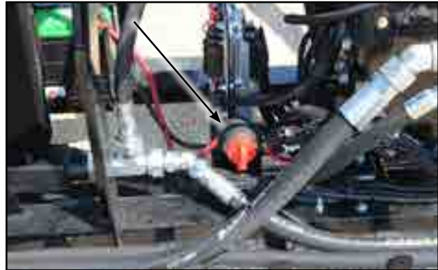
Fig 9 - Power shut-off switch
