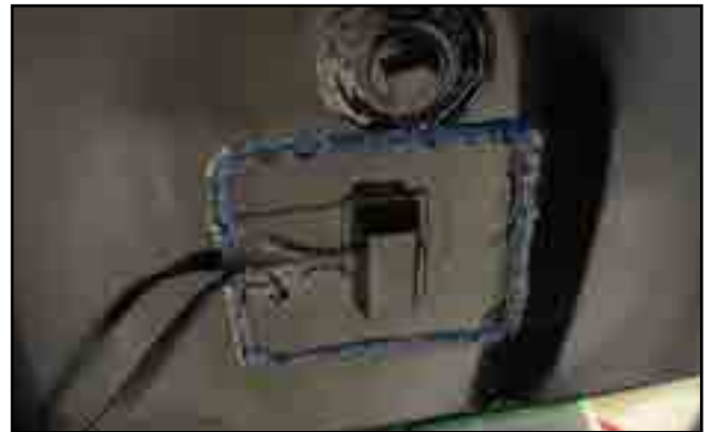
Fig 28 - Oil reservoir heater
